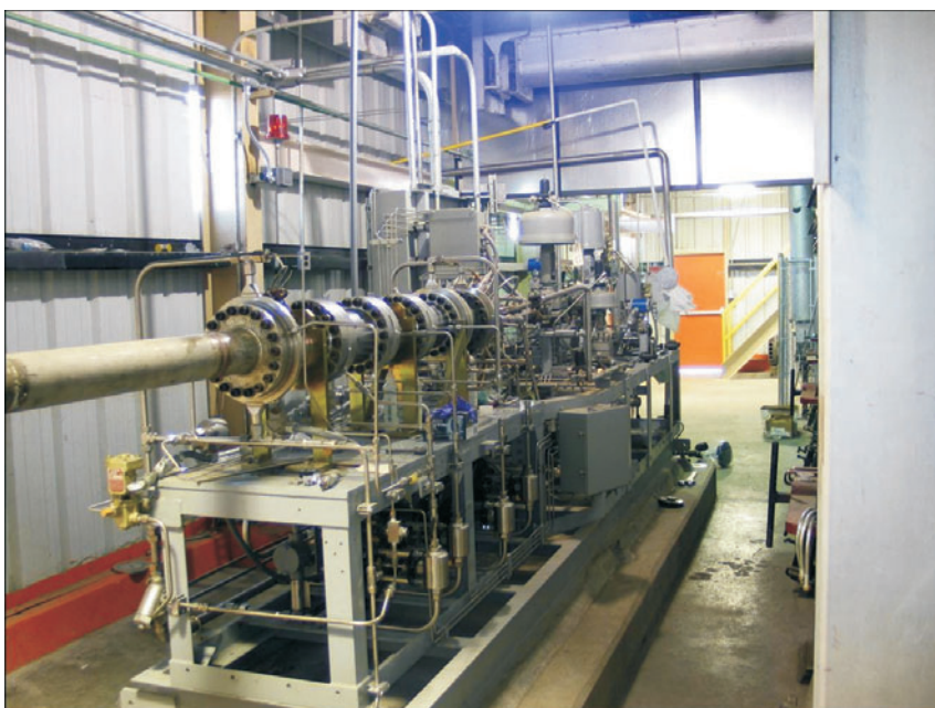
The gas generator at Kimberlina power plant. Natural gas and oxygen are combusted with recycled water to drive the turbines. (Image courtesy of CES)
