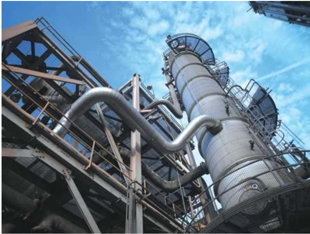
Integrated gasification combined-cycle power plants, like this one in Tampa, gasify the coal before combustion.
