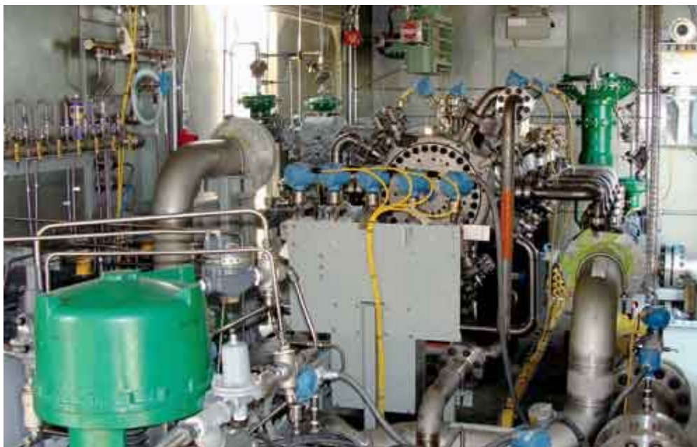
This oxy-fuel system manufactured by California-based Clean Energy Systems is ready for start-up. The injector (top) mixes fuel, oxygen, and diluent into the combustion chamber of the 200 MW thermal machine.
