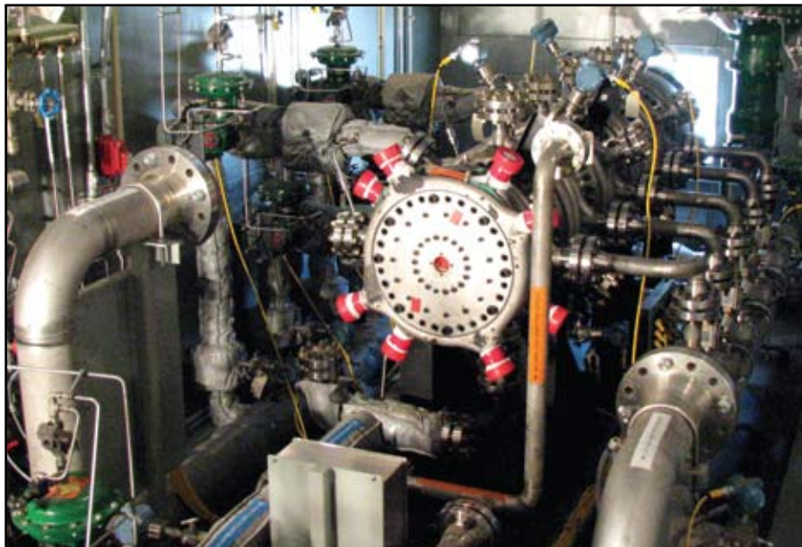
Oxy-fuel gas generator. Production unit is being readied for commissioning tests at the Kimberlina facility in preparation for the 50-MW WestCarb project installation. This oxy-fuel gas generator has a rated power level of 170 MWt on natural gas. It is about 100 inches long and 12 inches in diameter.
