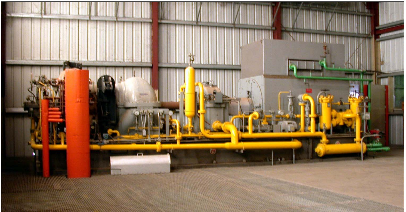
5.5 MW Steam Turbine and Generator
